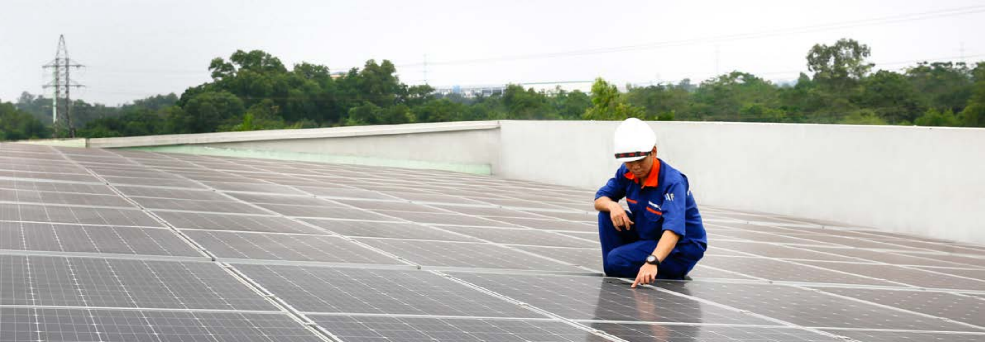
Photovoltaic cells of Vicostone's solar power system
