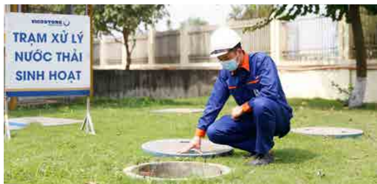
Wastewater treatment station
