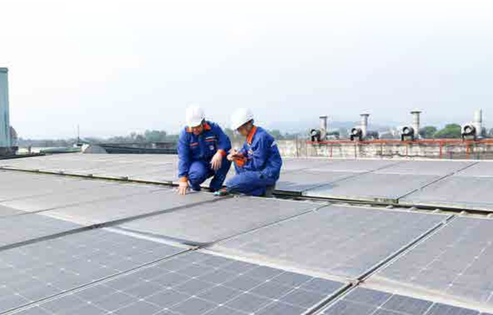
Solar power system
