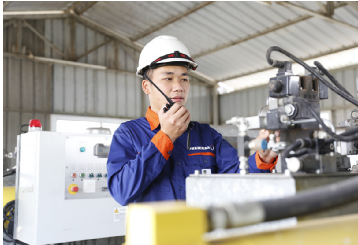
Fuel system under daily supervision by Vicostone's technicians
