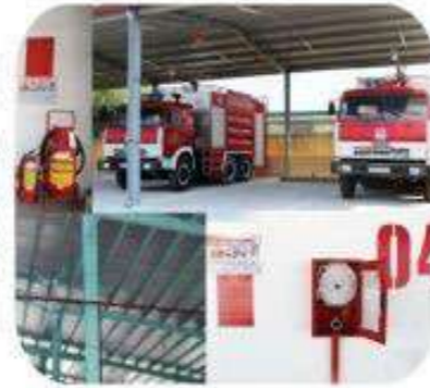
FIRE FIGHTING EQUIPMENTS
