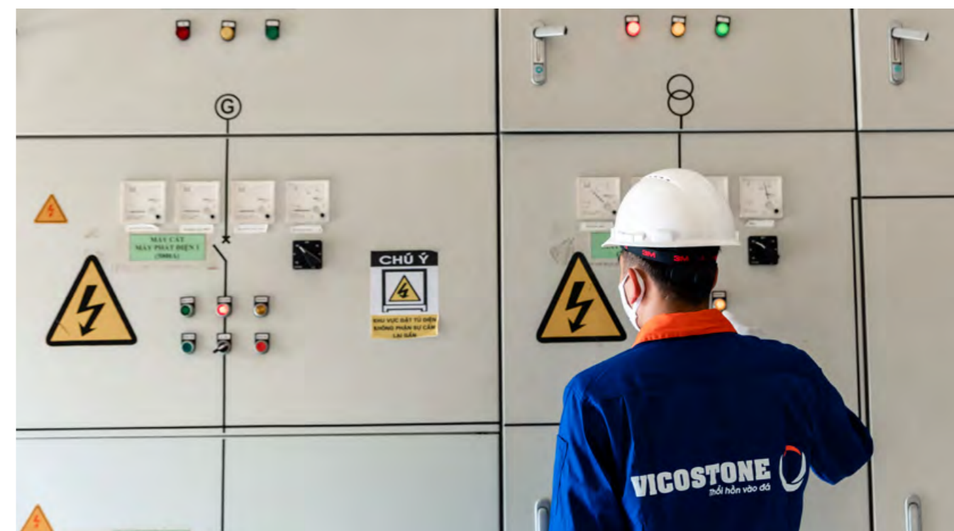
Engineers examine the electricity system on a frequent basis to ensure safety
