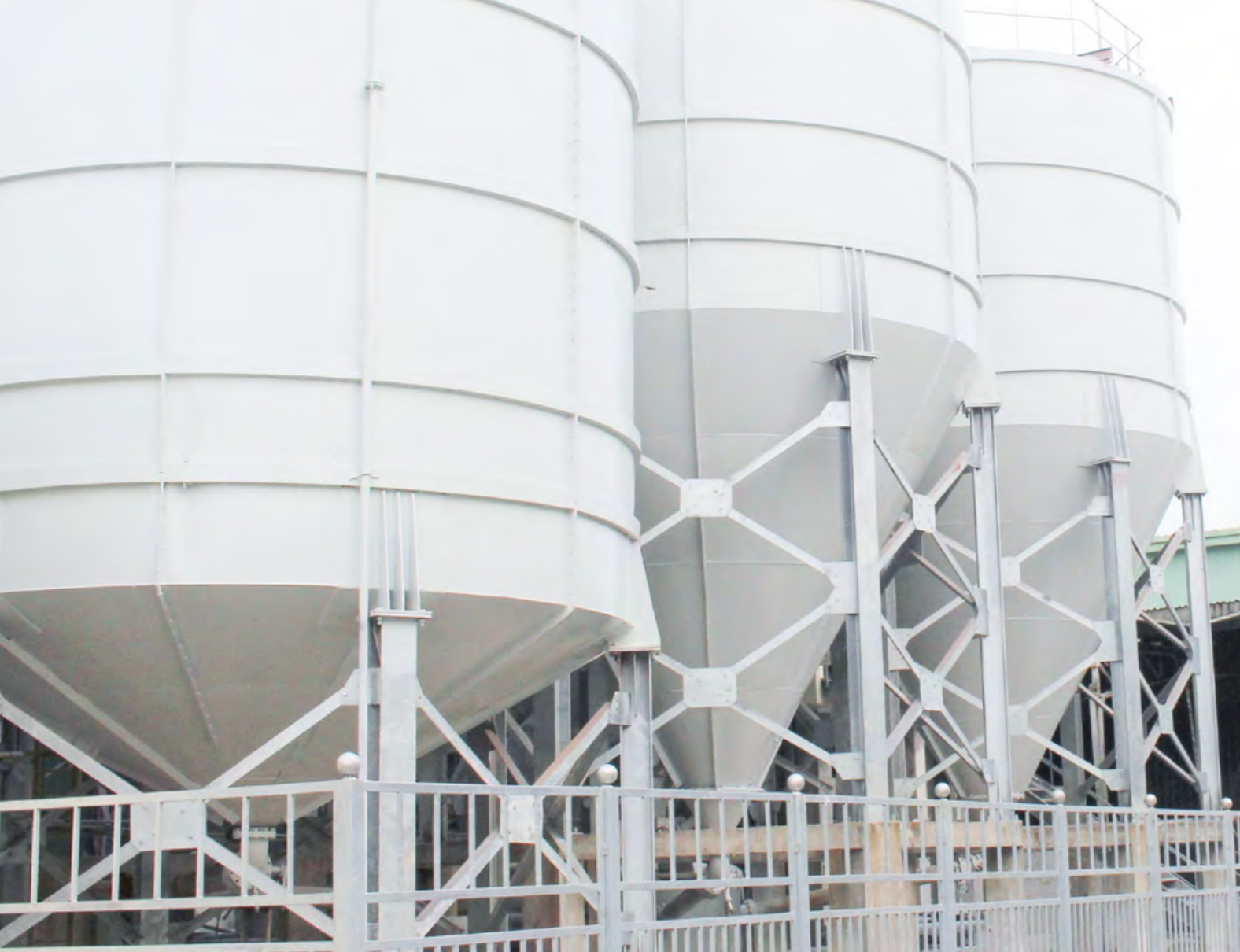
The silos used in water treatment at Vicostone
