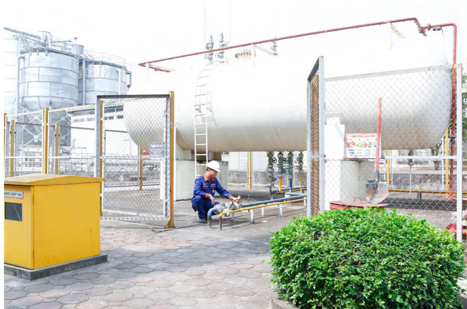
The gas supply system is periodically checked to ensure safety
