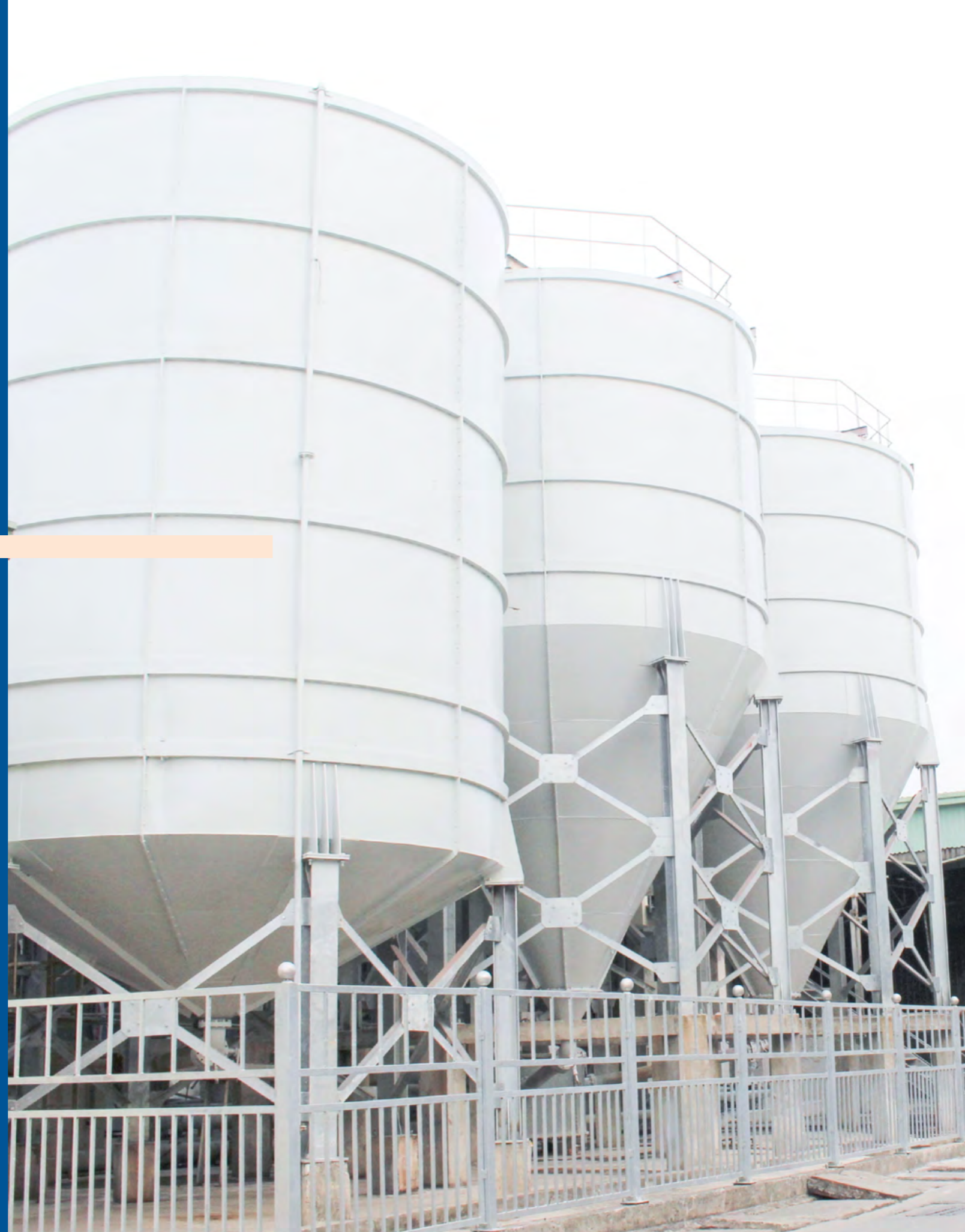
The silos used in water treatment at Vicostone
