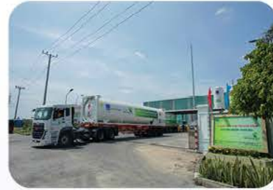
LNG satellite station at Thuan Dao Industrial Park, Long An
