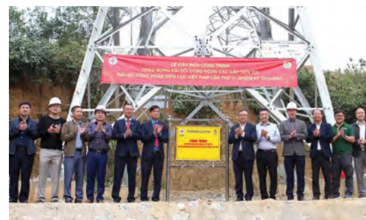
220kV Nam Mo - Tuong Duong transmission line project (section in Vietnamese territory)
