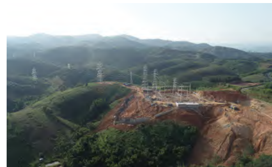
220kV Bo Y Substation and 220kV connecting transmission lines
