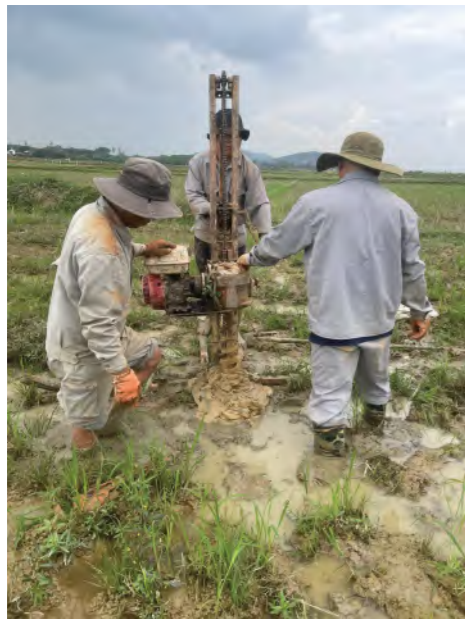
Geological survey for the 200kV transmission line connecting the Truong Son wind power plant (Laos) to Do Luong Substation (section in Vietnamese territory)
