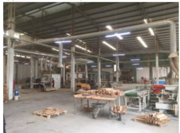
Modern Dust Extraction System
