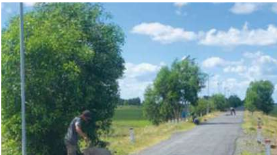
Solar Lighting at Long An Border with Cambodia
