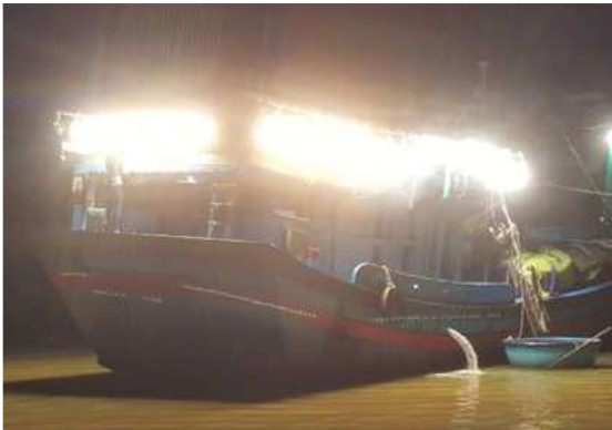
LED Fishing Light Installation in Quang Ninh
