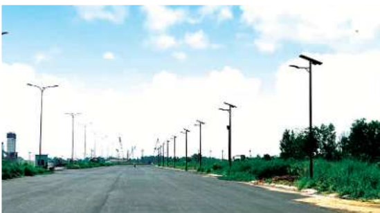
Solar Lighting at Aquacity Urban Area - Long Hung - Bien Hoa
