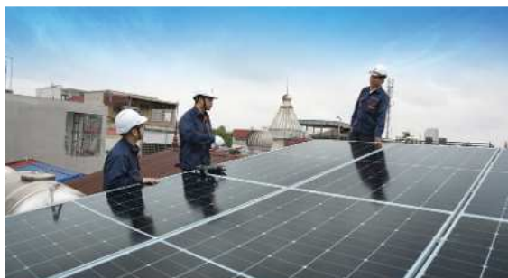
Roof-top Solar Lighting in Hai Phong
